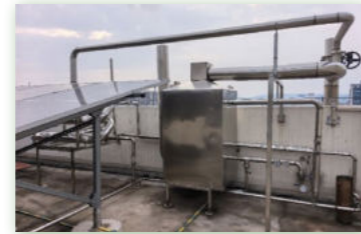
Flash Steam Recovery System at Xiang Peng Plant
