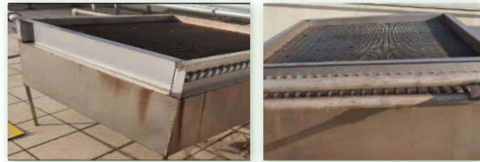
Steam Emission and Condensate Heat Recovery Equipment at Hua Peng Plant Shrink Tunnel
